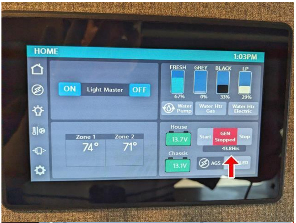
16.18 Item 5 (Picture) Generator Hours = 43.8
