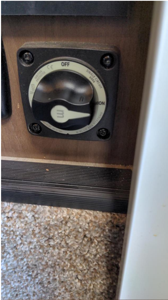
16.12 Item 1 (Picture) battery disconnect switch
