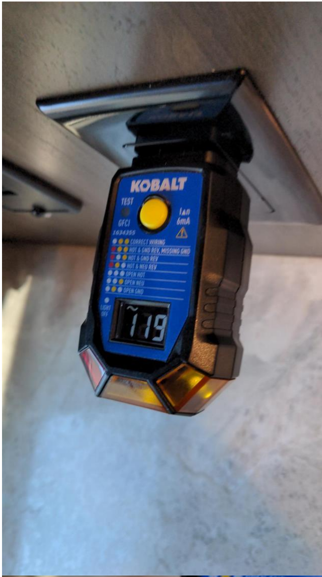
16.15 Item 1 (Picture) Bedroom 120 VAC Outlet
