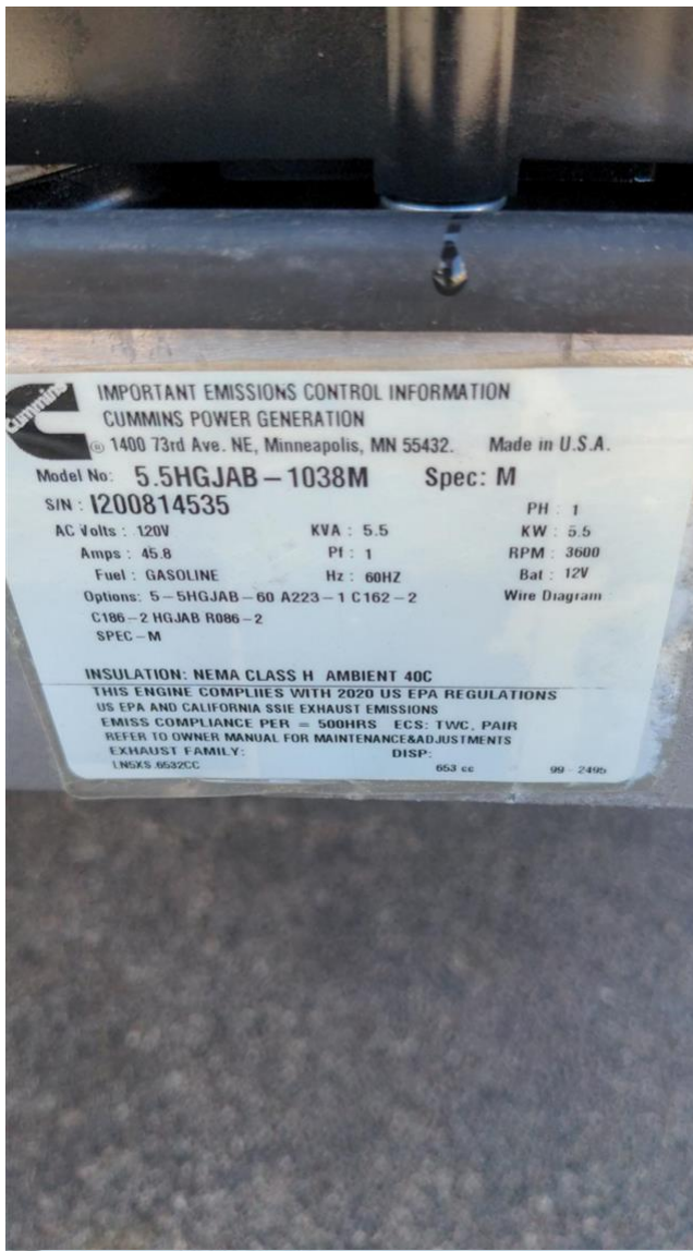
16.18 Item 3 (Picture) generator data plate
