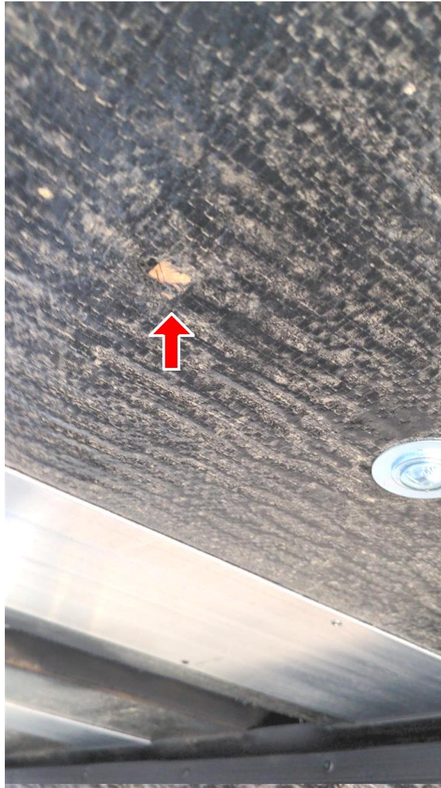
12.3 Item 2 (Picture) slide out floor small defect
