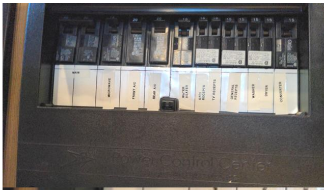
16.3 Item 1 (Picture) electrical panel boxelectrical panel box
