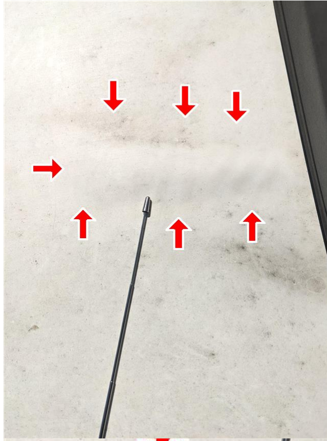
17.0 Item 3 (Picture) Bubble in roof membrane
