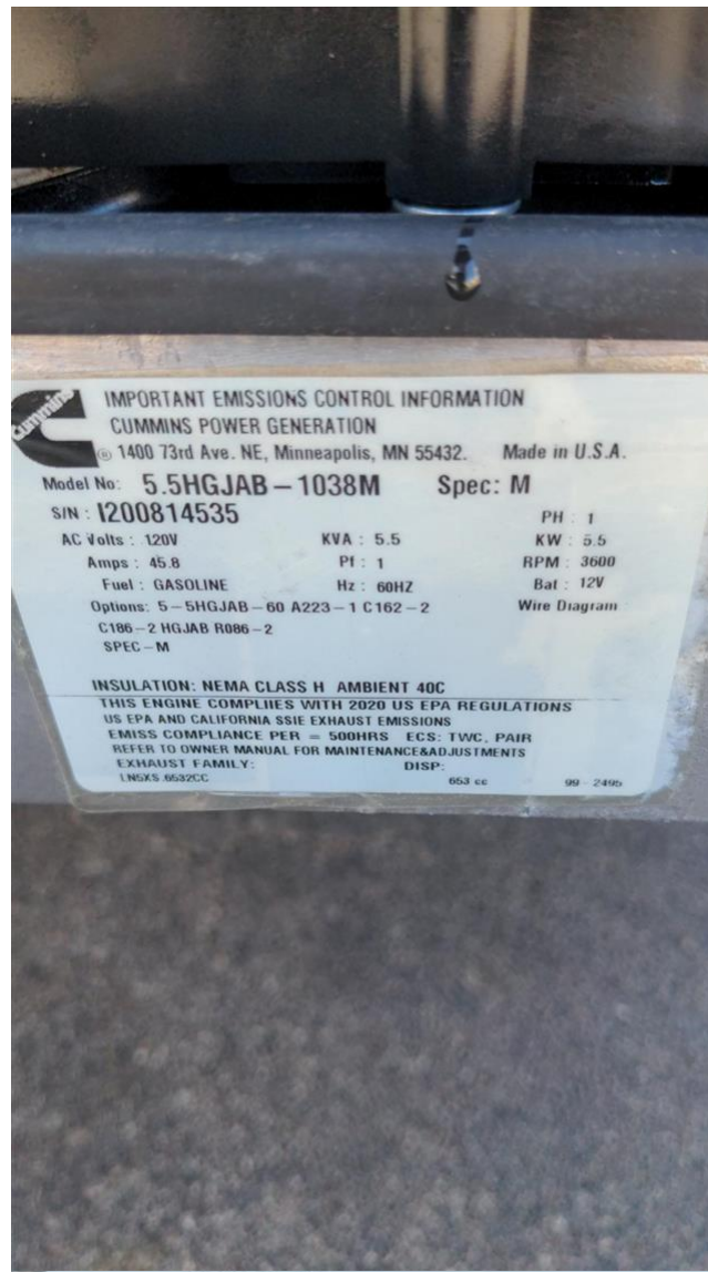
16.18 Item 3 (Picture) generator data plate
