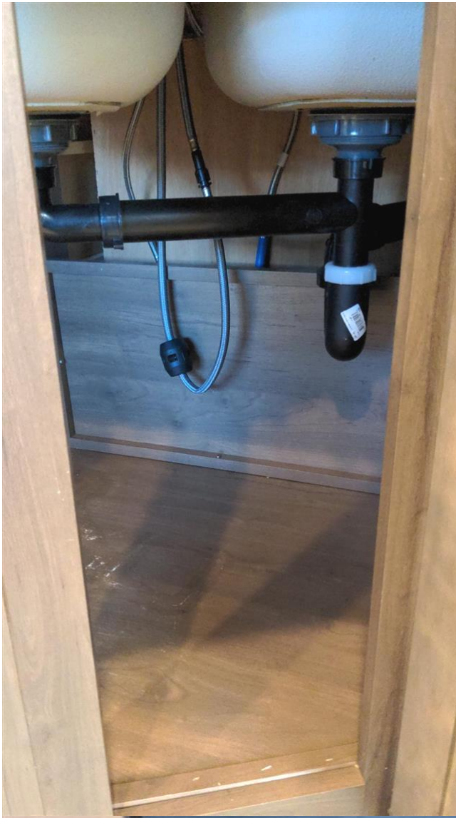
20.2 Item 1 (Picture) kitchen sink plumbingkitchen sink plumbing
