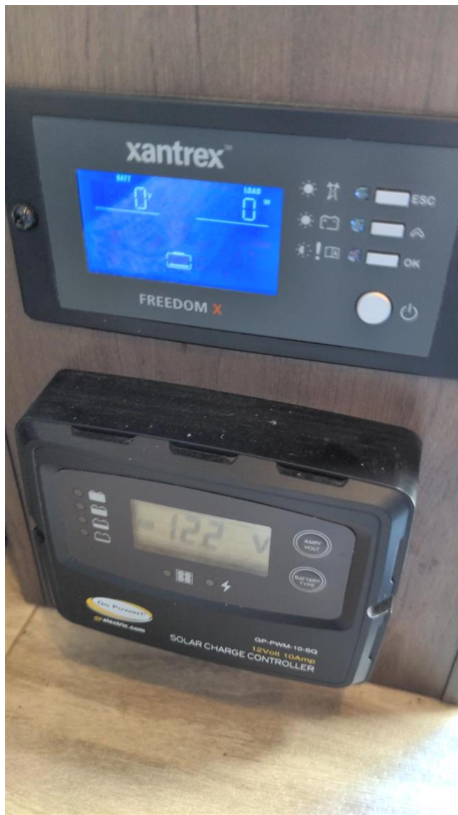
16.20 Item 1 (Picture) solar charge controller
