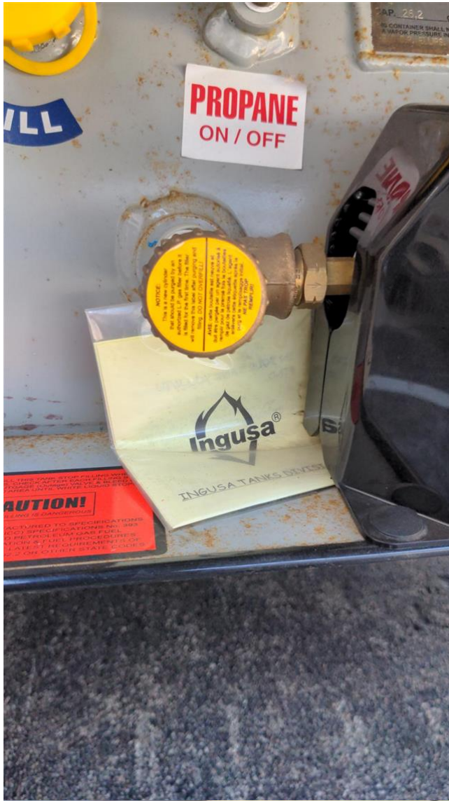
15.2 Item 1 (Picture) propane shut off valve
