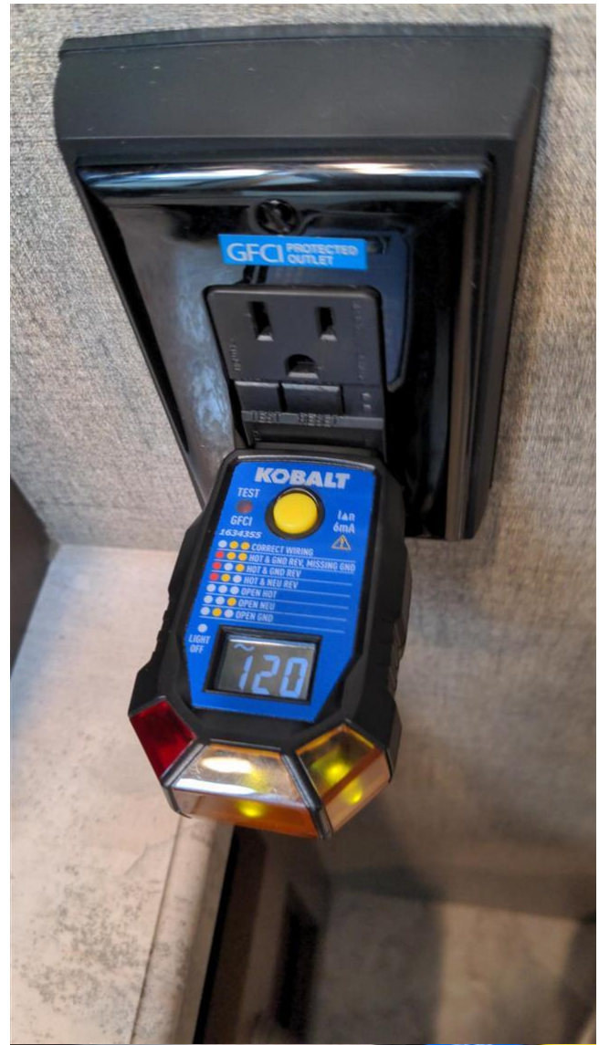
16.1 Item 2 (Picture) bathroom outlet
