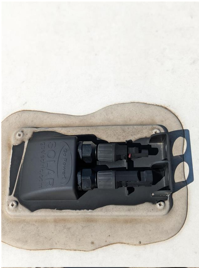
17.15 Item 1 (Picture) Solar Controller
