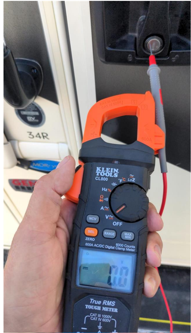
2.2 Item 2 (Picture) door voltage
