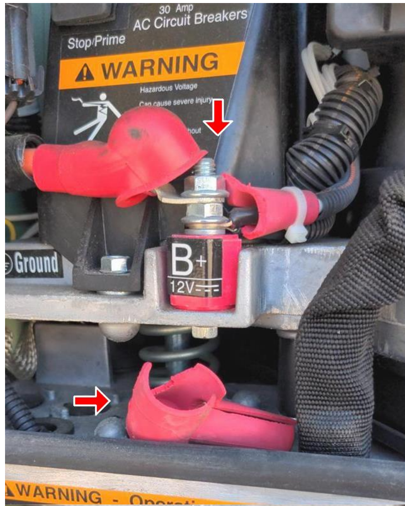
16.18 Item 1 (Picture) damaged electrical power covers
