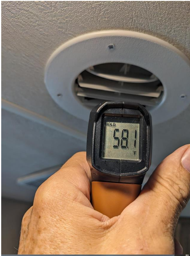
21.0.A Item 1 (Picture) AC temperature
