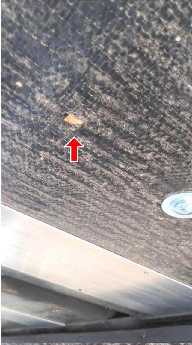
12.3 Item 2 (Picture) slide out floor small defect
