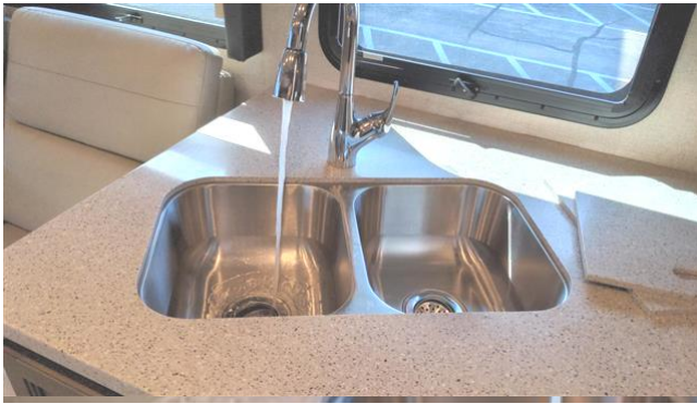
20.0 Item 1 (Picture) overview of kitchen plumbing
