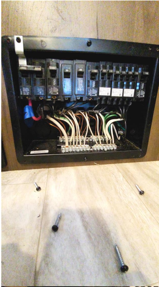
16.3 Item 2 (Picture) electrical panel box wiring
