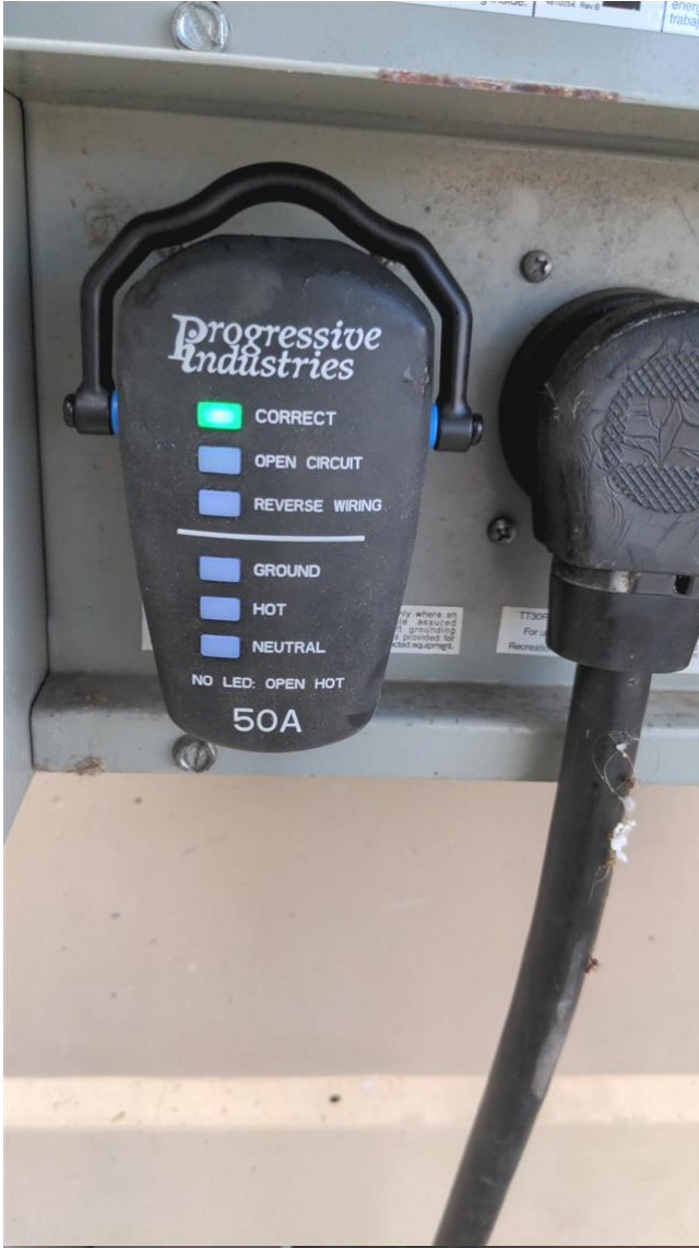
2.1 Item 1 (Picture) Shore Power Outlet Polarity
