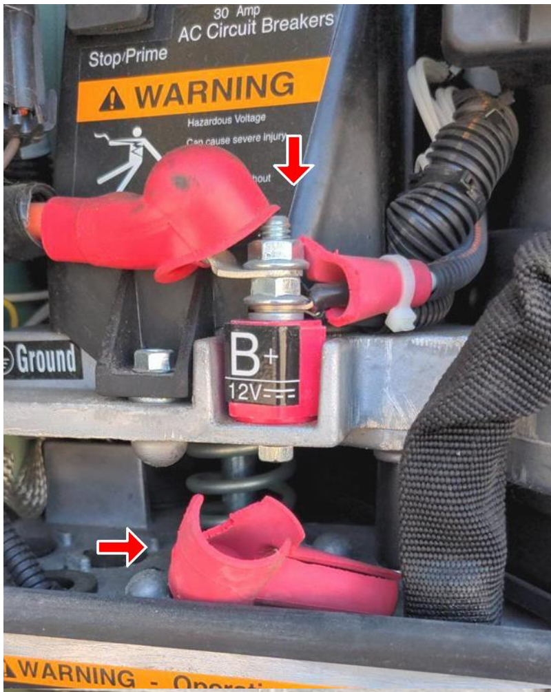
16.18 Item 1 (Picture) damaged electrical power covers
