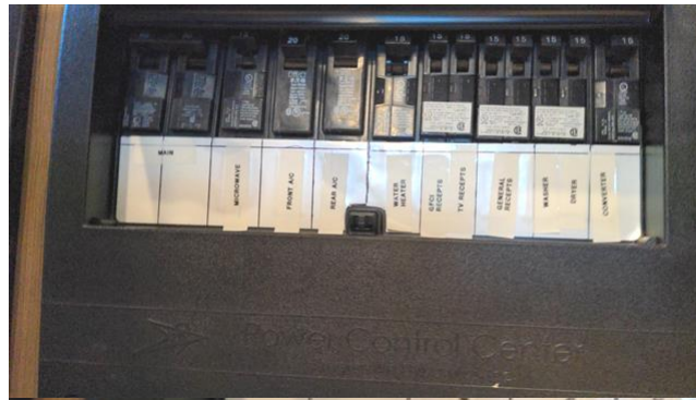
16.3 Item 1 (Picture) electrical panel boxelectrical panel box
