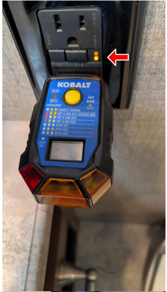
16.2 Item 2 (Picture) GFCI outlet tripped
