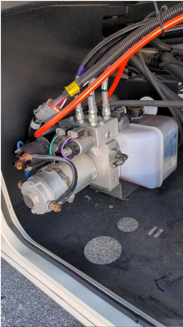
25.2 Item 1 (Picture) hydraulic pump in battery Bay
