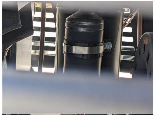
17.10 Item 2 (Picture) AC interior
