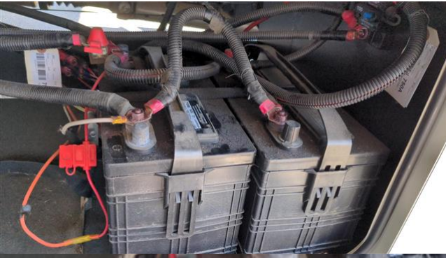
16.11 Item 1 (Picture) Coach batteries
