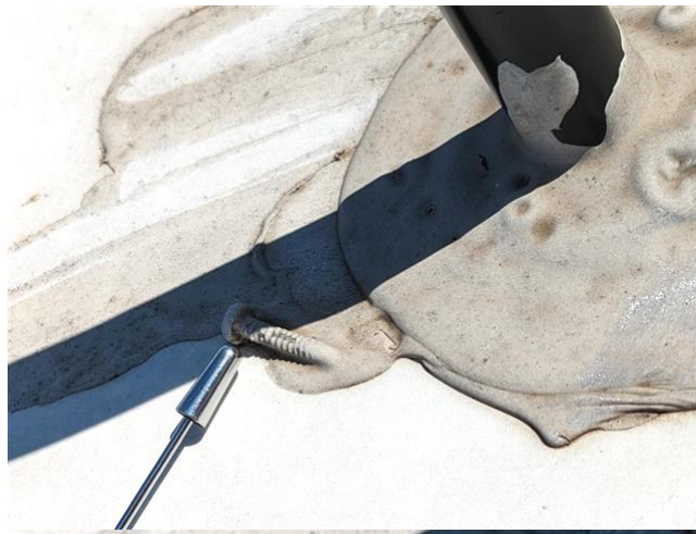
17.16 Item 3 (Picture) Screw in Sealant
