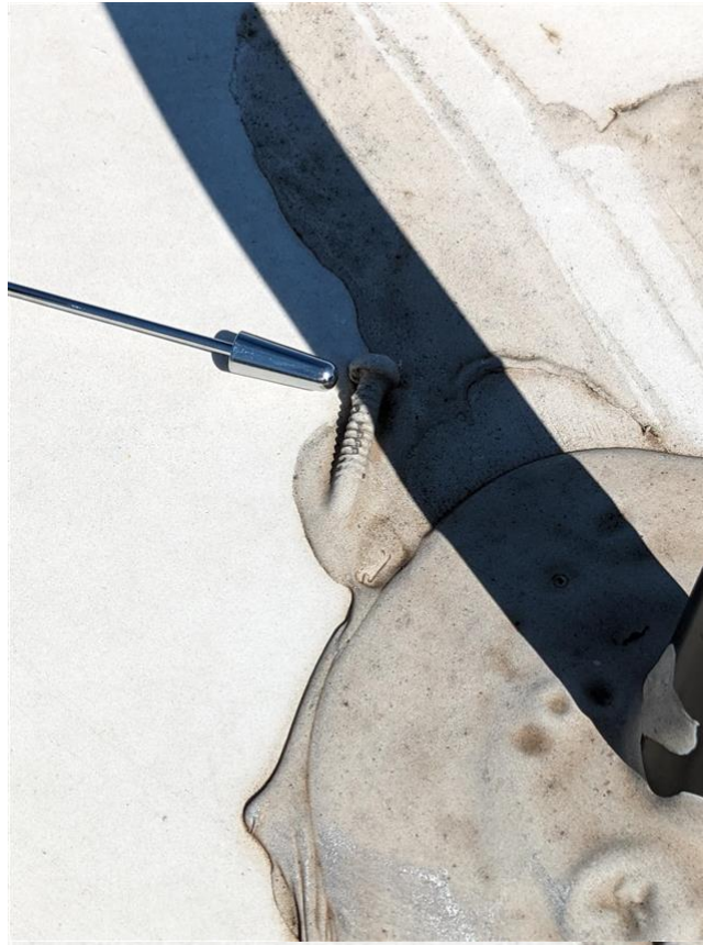
17.16 Item 2 (Picture) Screw in sealant
