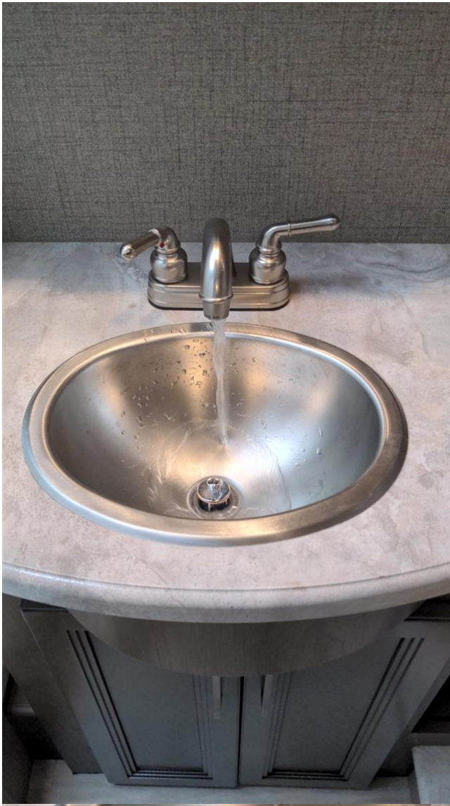
20.8 Item 1 (Picture) bathroom faucet
