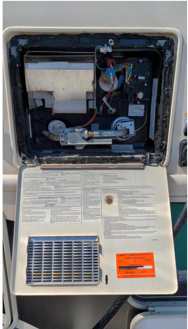
13.0 Item 2 (Picture) water heater cover open
