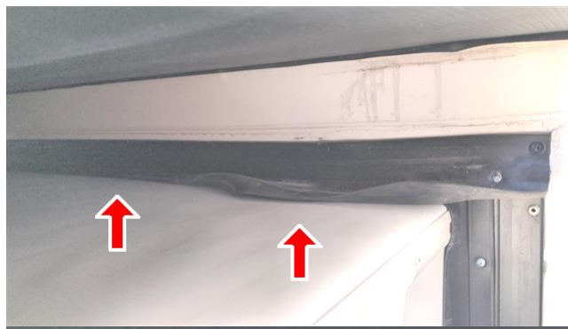
9.7 Item 5 (Picture) curbside slide out roof seal and sweep
