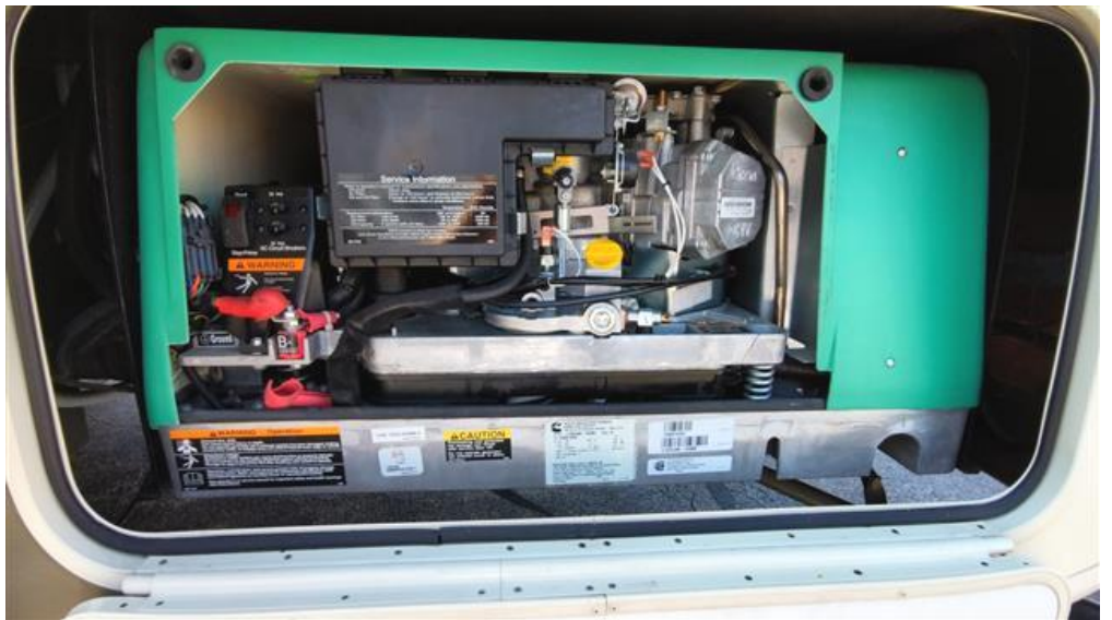
16.18 Item 2 (Picture) overview of generator
