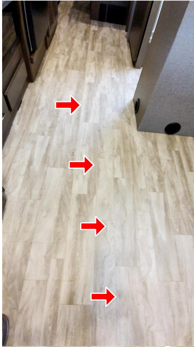
22.19 Item 1 (Picture) floor scratch
