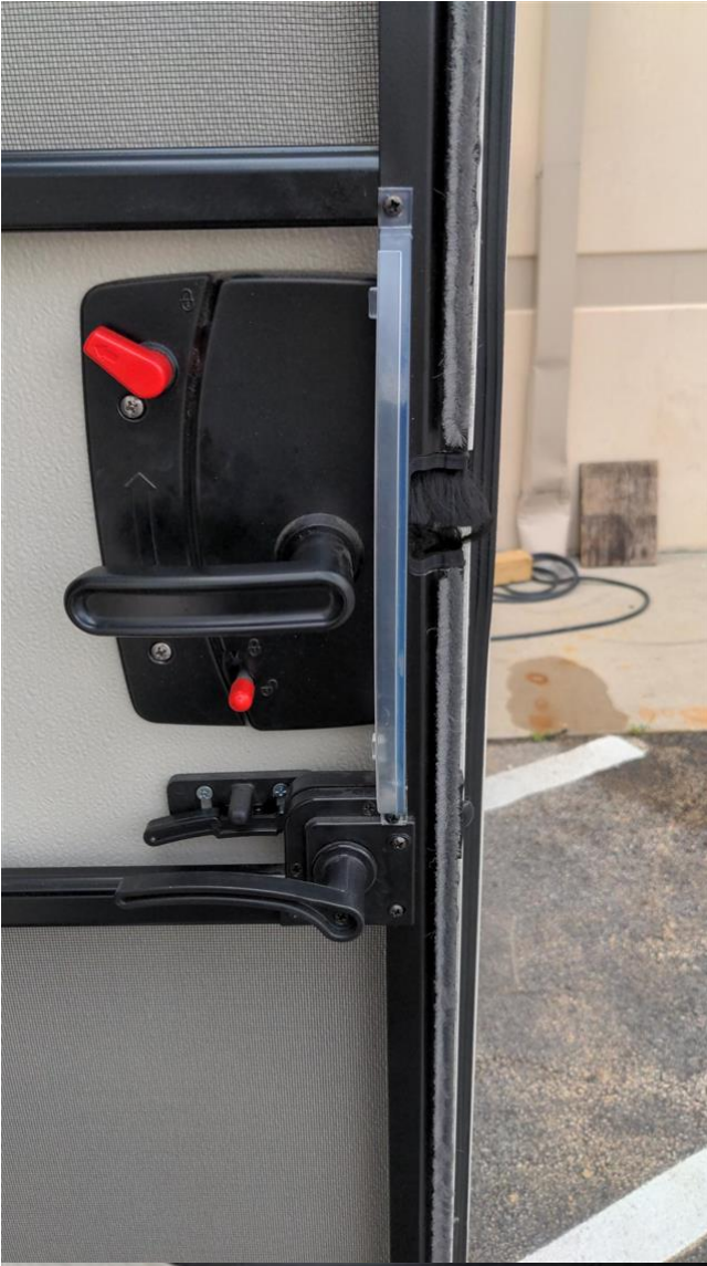
6.7 Item 1 (Picture) door deadbolt lock open
