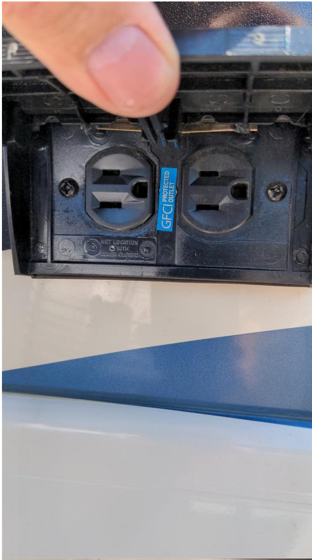
16.14 Item 1 (Picture) external 120 volt outlets
