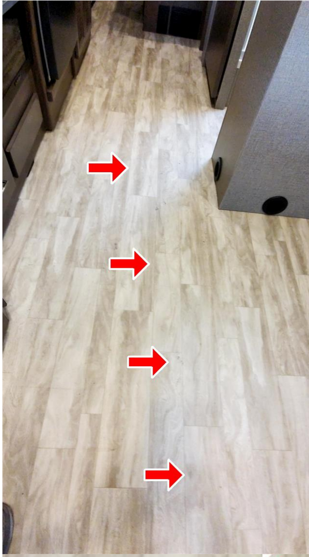
22.19 Item 1 (Picture) floor scratch
