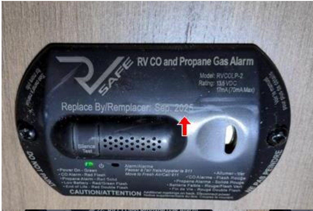
19.1 Item 1 (Picture) LP/CO detector expires September 2025
