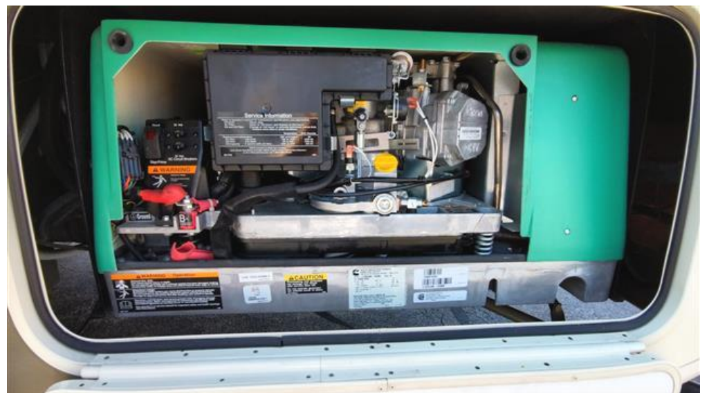
16.18 Item 2 (Picture) overview of generator
