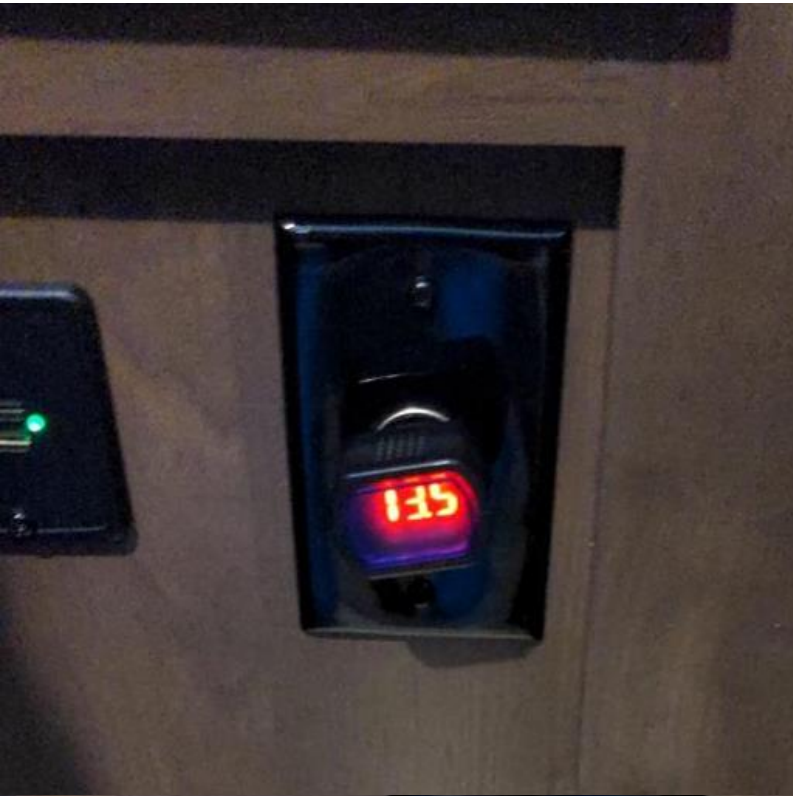
16.16 Item 2 (Picture) 12 volt receptacle voltage
