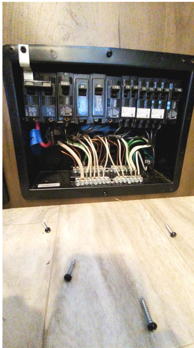
16.3 Item 2 (Picture) electrical panel box wiring
