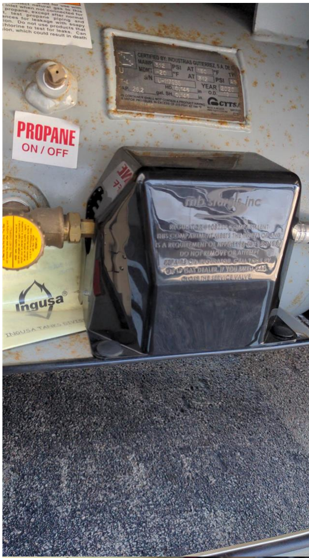
15.1 Item 1 (Picture) regulator inside cover
