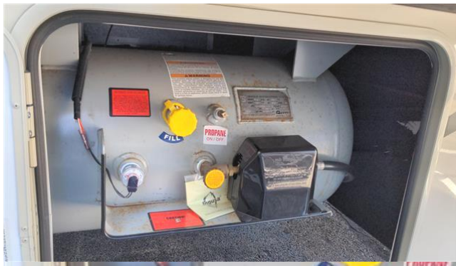
15.0 Item 1 (Picture) ASME tank overview
