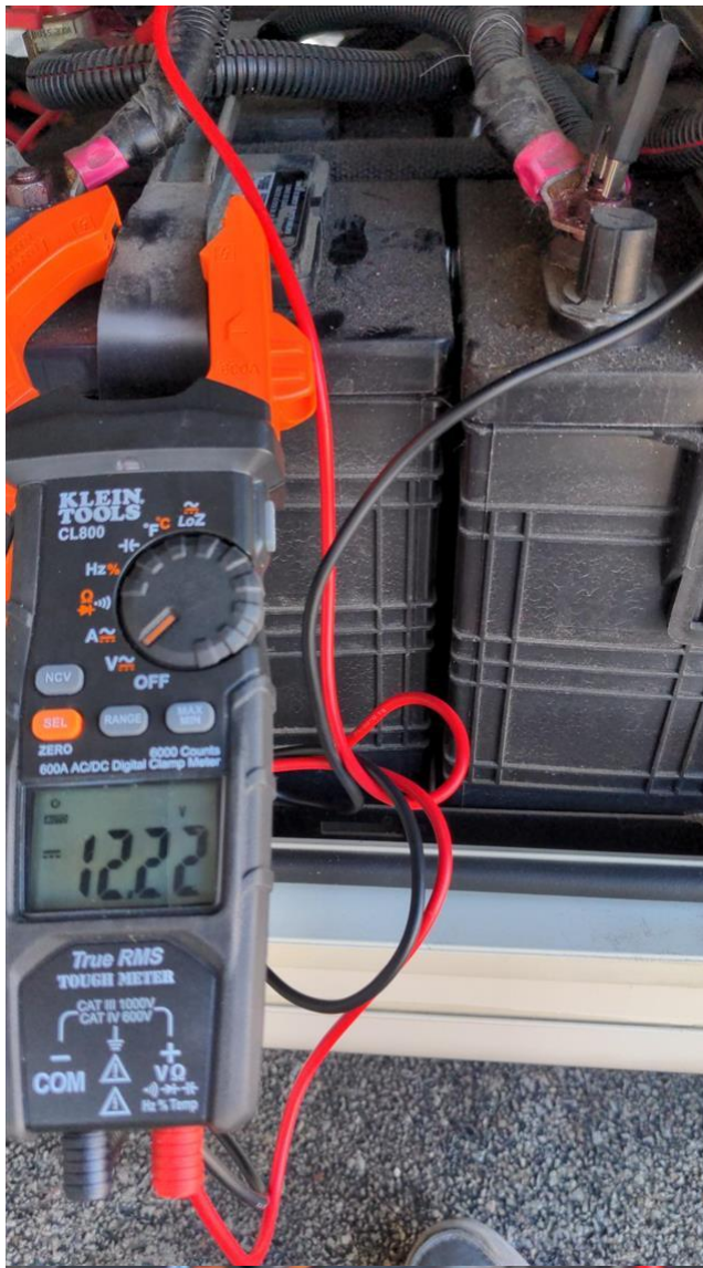
16.6 Item 2 (Picture) battery voltage external power off
