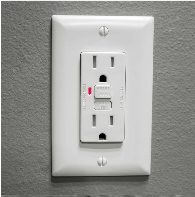
16.2 Item 1 (Picture) Typical GFCI Outlet
