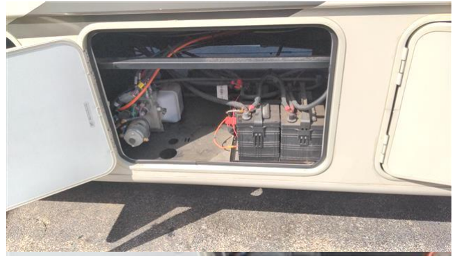
11.5 Item 5 (Picture) electrical bay
