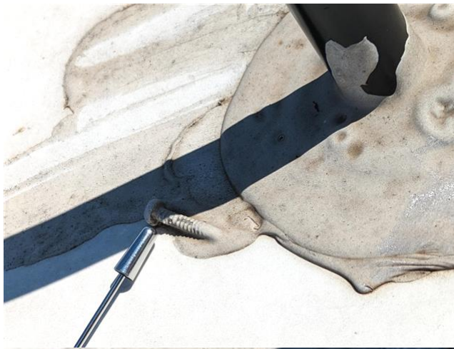
17.16 Item 3 (Picture) Screw in Sealant
